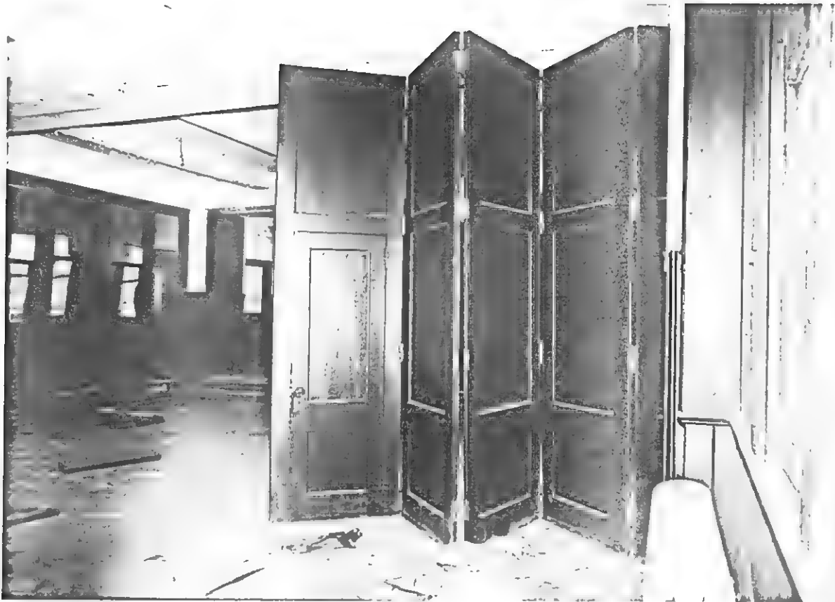
Wooden sliding doors are intact in the stepped second floor of the YMCA Building auditorium/lunchroom.
